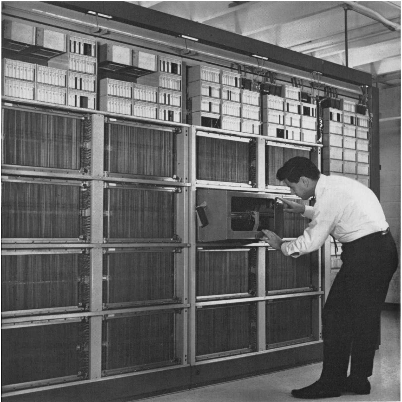
The program store modules of the Succasunna office of ESS. These 16 modules hold more than 5 million bits of information.
