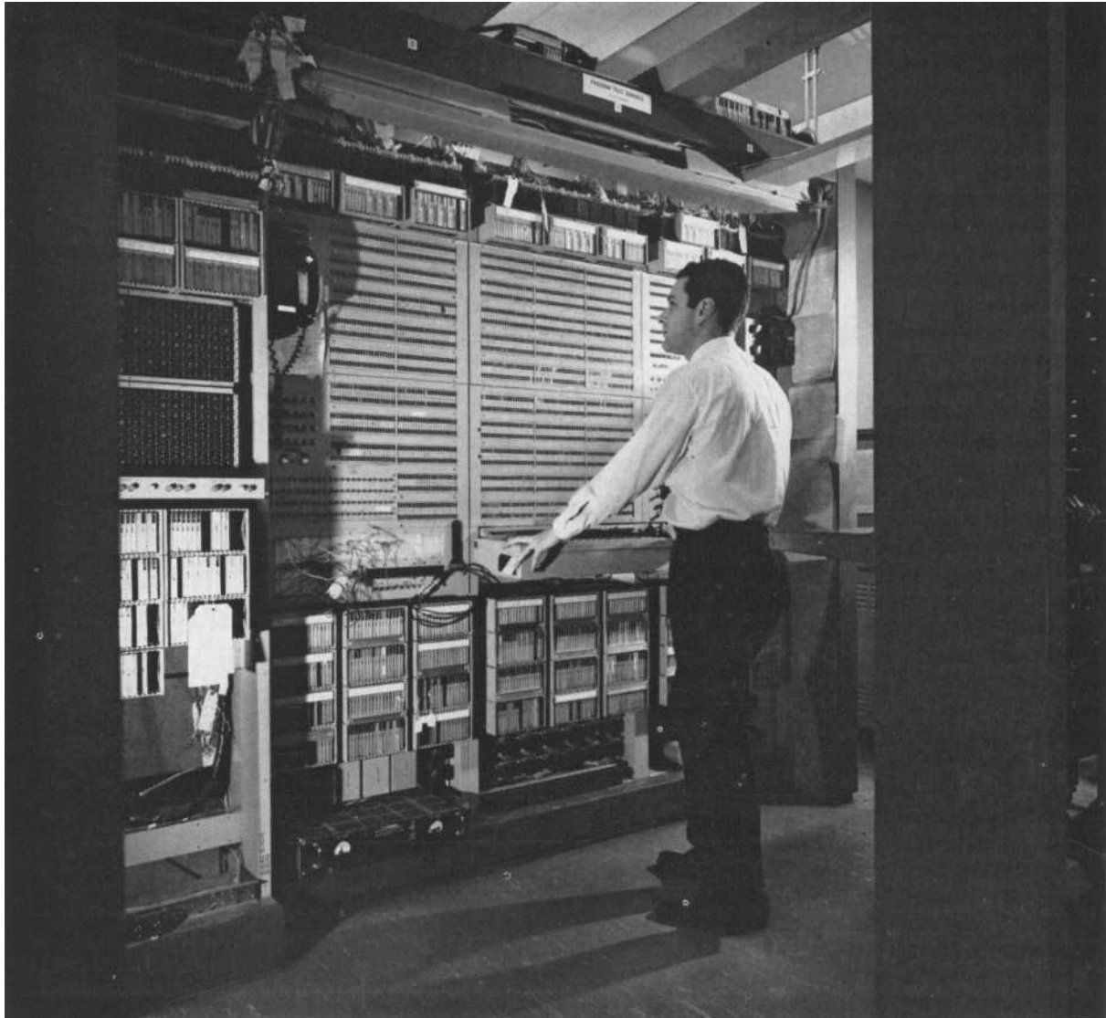
The author studies lamp indications on the program test console of the Holmdel Laboratory No. 1 ESS. This console simultaneously monitors 864 points in each central control. The parallel strips display the state of twin points in each control.
