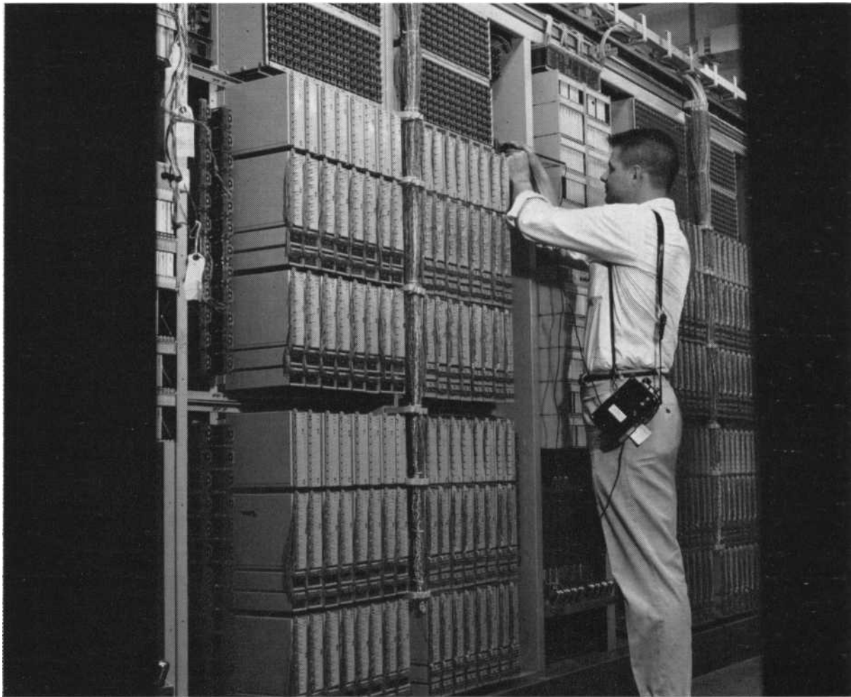
J. Bodirae, a Western Electric craftsman, performs an installation test on line switching frames.
