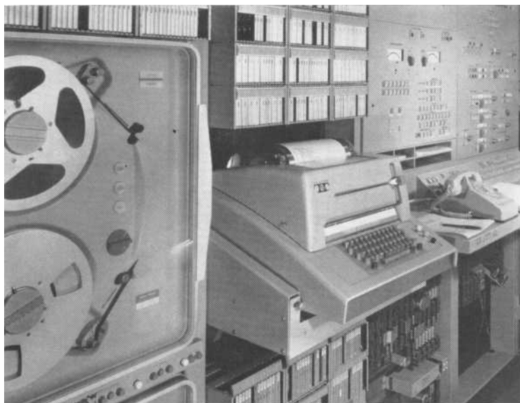
The master control center at the Succasunna No. 1 ESS office. Controls and lamps on the panels at the far right are used for various maintenance and administrative functions. The teletypewriter supplements the panel controls. The tape reels at the left are used for automatic message accounting recordings.
