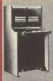
Answering Service Switchboard — used to intercept calls to business or professional people who are out of their offices.
