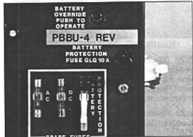
FIGURE 14—MPSA CONTROL PANEL
